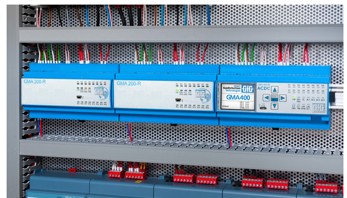
GMA400 with two relay modules GMA200-RT in the control cabinet structure
