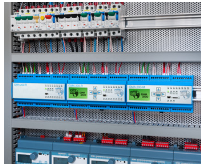
GMA200-MT with two relay modules GMA200-RT and GMA200-RTD mounted in a control cabinet.
